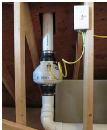
EXAMPLE OF RADON BLOWER MOTOR
